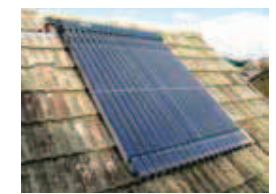
solar thermal panels for hot water
