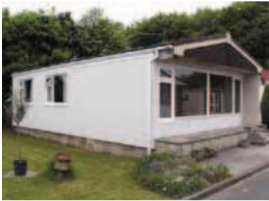
External Wall Insulation on a property in Bath & North East Somerset undertaken as part of the Council's Freedom from Fuel Poverty Project
